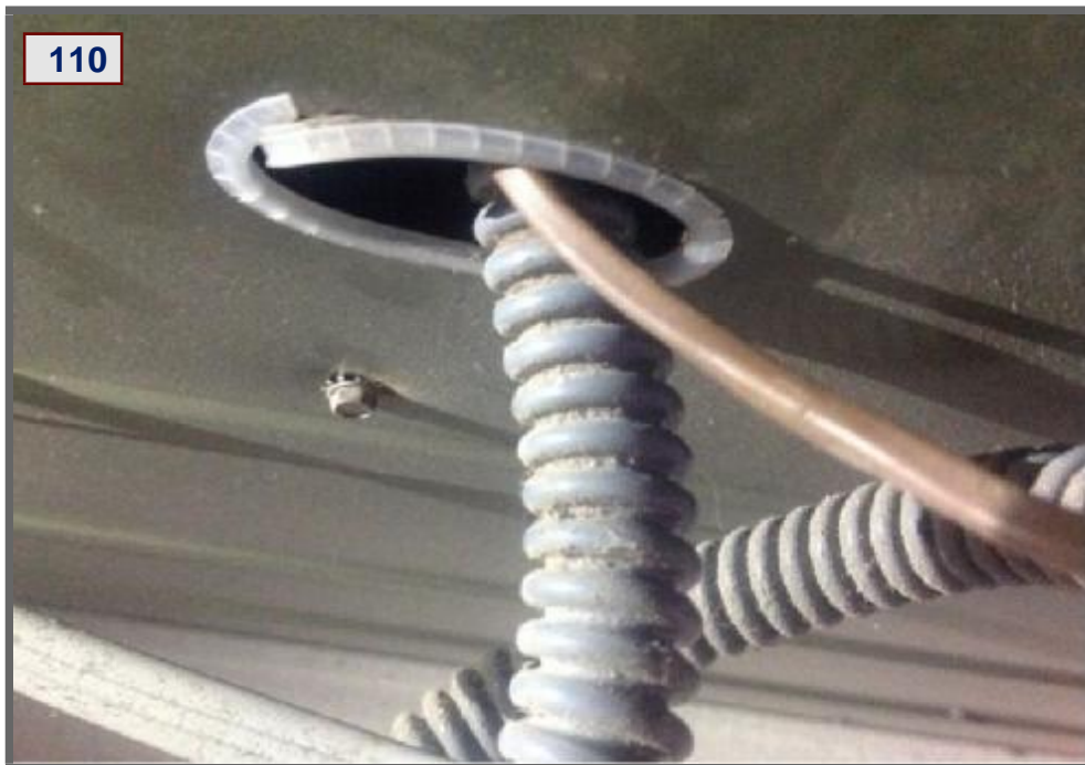
Gas Line In Properly Installed
