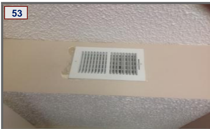
Damage Noted at Vent
