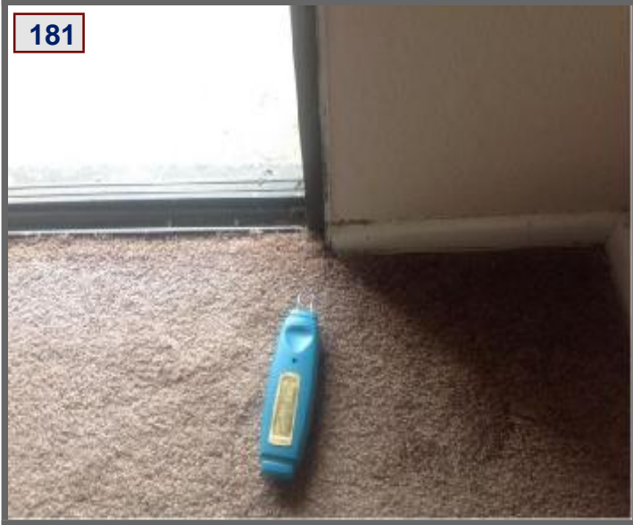
Right side of Sliding Door Moisture Noted (2)
