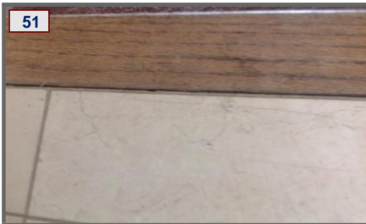
Danger: Trip Hazard, Hall Entry To Down Stairs
