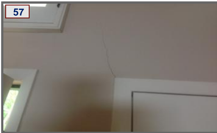
Crack at Enter hall Above Garage Entry Door
