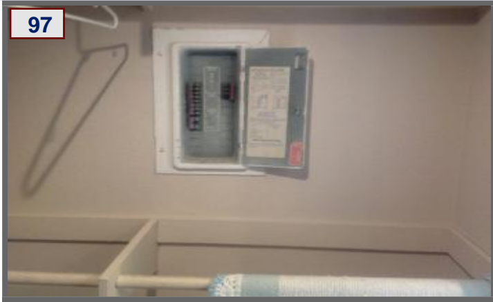
Main Electric Panel
