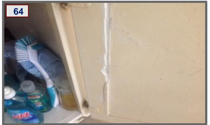
Water stain on Kitchen Window Seal and wall
