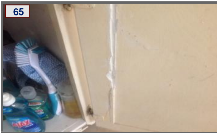
Damage to Kitchen Sink Cabinet
