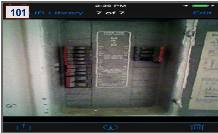
Electric Main Panel In Closet , No Hot spots Noted
