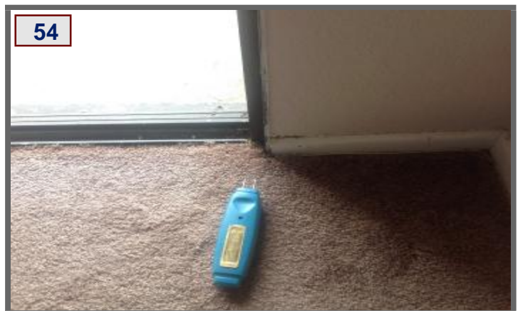
Moisture Noted in Carpet at sliding Door Bedroom 2
