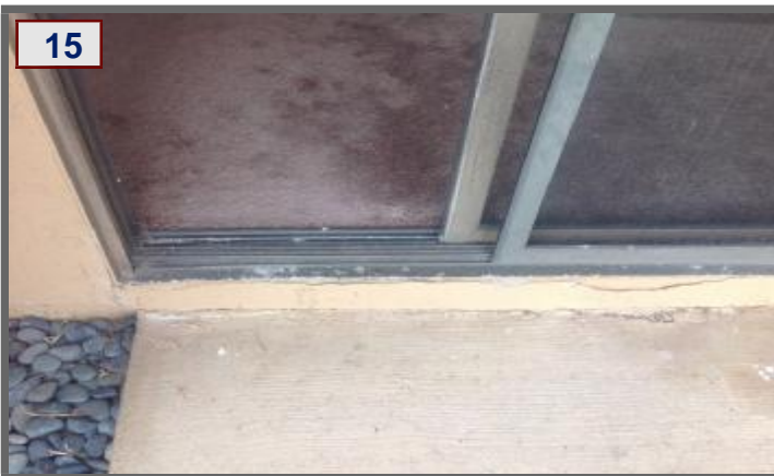
Exterior Stucco Damage
