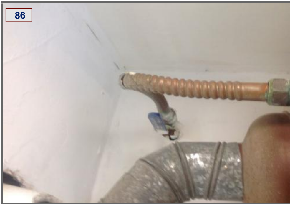
Hot Water Heater Shut off Valve Corroded
