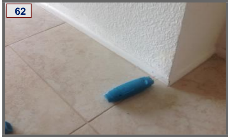
Kitchen in Wall Moisture Noted With Moisture Probe
