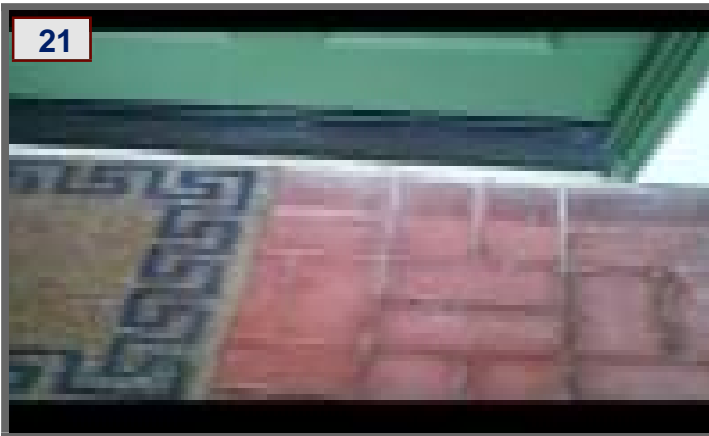
Front Entry Exterior Moisture Noted Recommend to Redirect Watering
