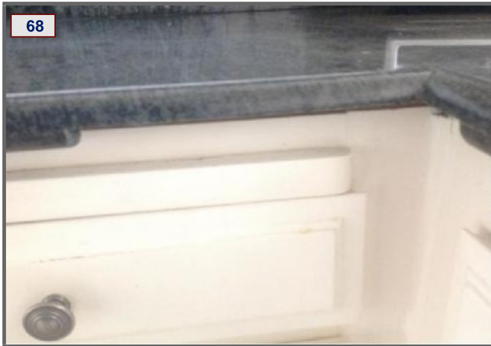
Damaged Garnet at next to Kitchen Sink
