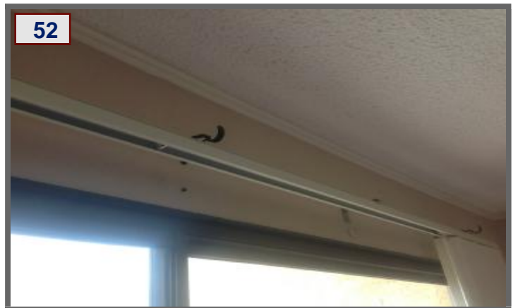
Bedroom 2: Wall above Sliding doors Needs Repair
