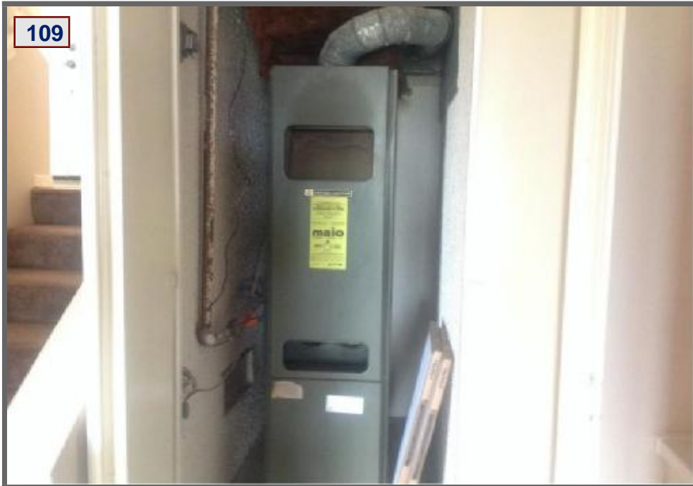
Heater Located in Closet
