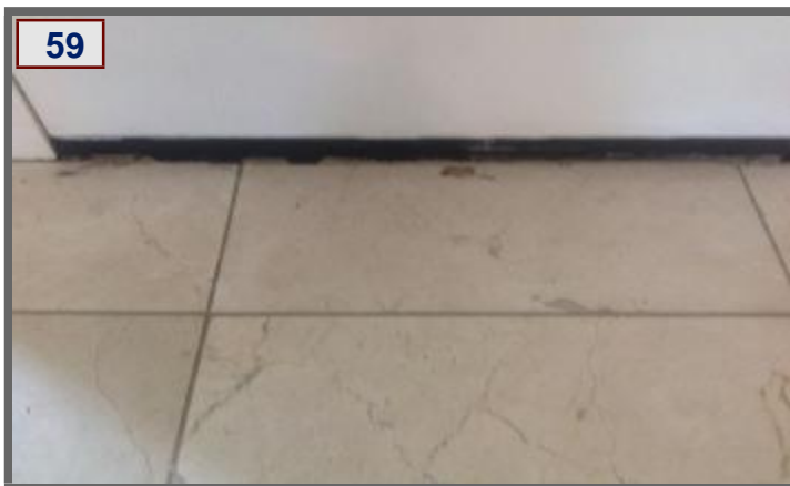
Damaged Floor at Garage Enter Door
