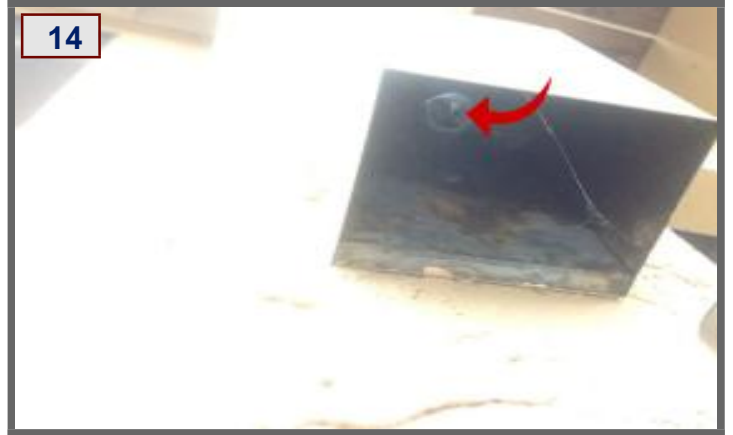
Exterior Light Damaged
