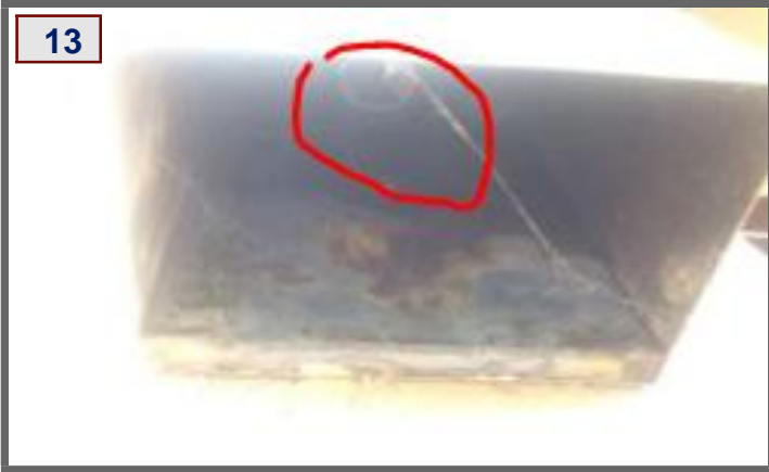
Exterior Light Damaged
