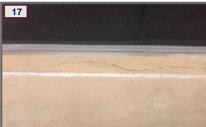
Exterior Stucco Damage
