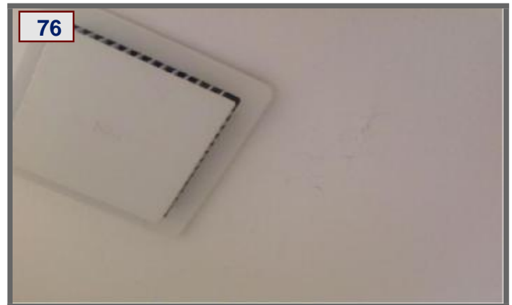
Entry Hall 1/2 Bath Exhaust Fan needs Repaired/Replaced
