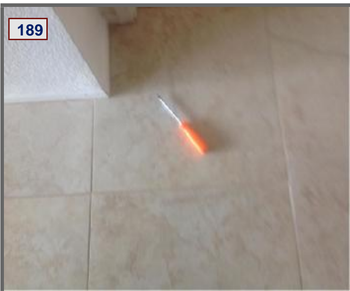
Loose Tile And Moisture Noted
