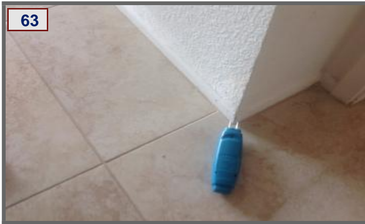
Kitchen in Wall Moisture Noted With Moisture Probe , Kitchen in Wall Moisture Noted With Moisture Probe
