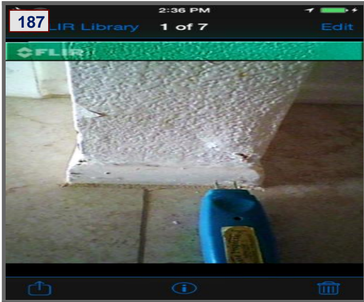
Kitchen Moisture Noted in Several Areas
