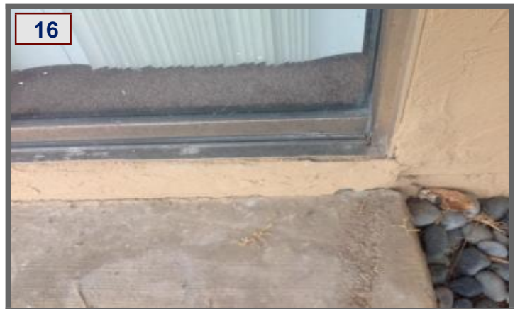
Exterior Stucco Damage
