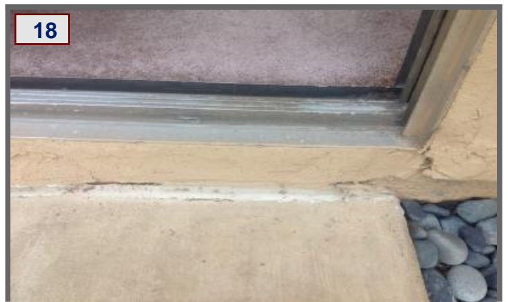
Exterior Stucco Damage
