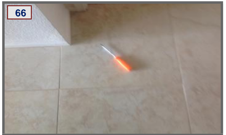
Kitchen Tile Not sealed to Floor
