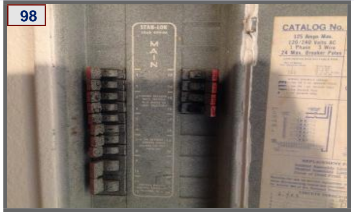
Main Electric Panel
