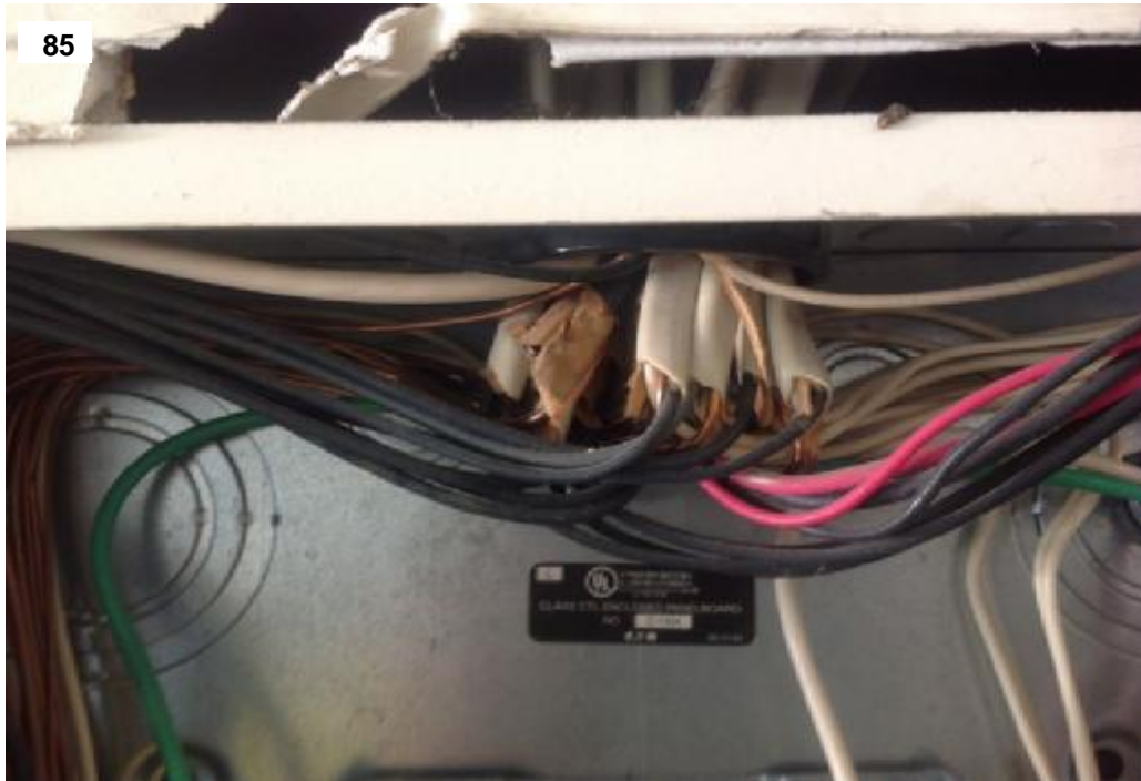
Conductor wires entering one knockout
