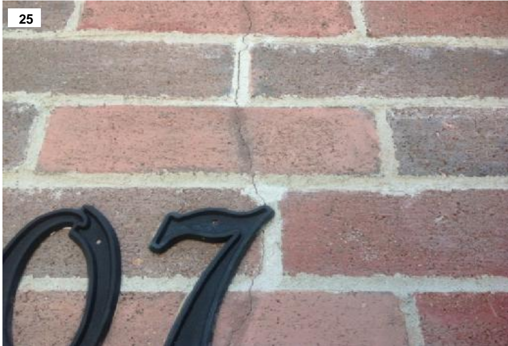
Crack in brick veneer located above garage
