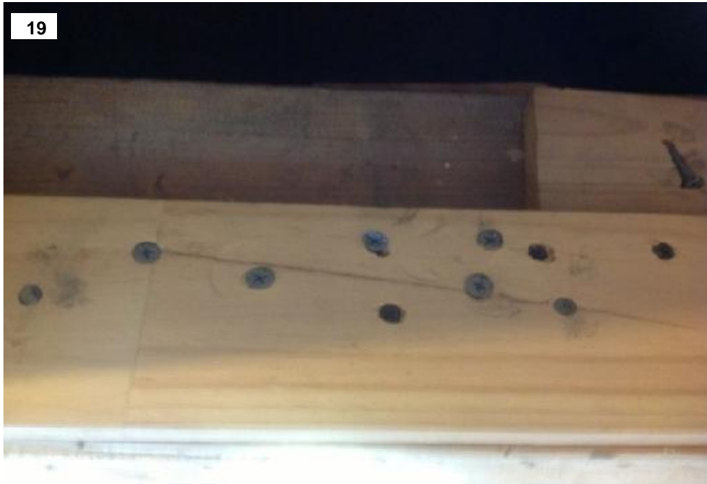
improper attachment of pull down stairs
