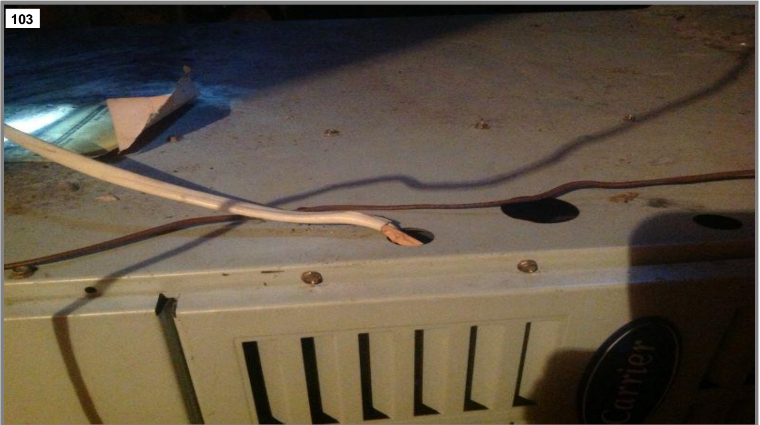
Unprotected wire going into furnace
