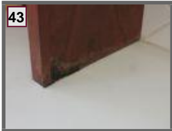
Hall Entry Door Water stain
