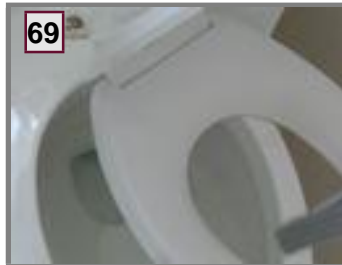
69 Master Bathroom Toilet: Seat Needs Adjustment / repair required to Operate properly (2) See Photo # 69
