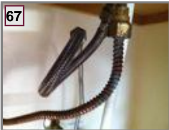
67 Master Bathroom Signs of past leaks/corrosion at drain lines under sinks. Noted Micro leek (2) See Photo # 67
