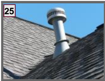
Shingles need secured & sealed at one or more locations.
