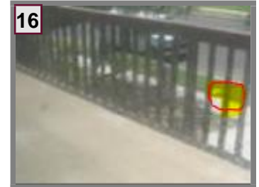
View of Exterior railing opening 7-8 inch
