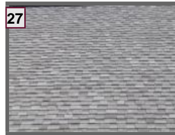
Shingles showing signs of weathering & age.
