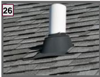
Shingles showing signs of weathering & age.
