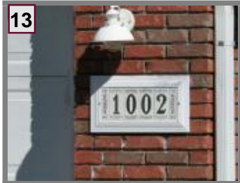
Front Light Bulb missing
