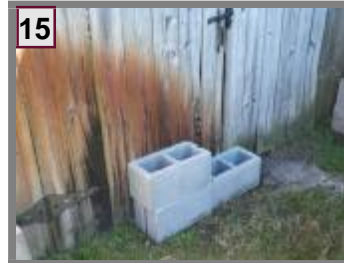
Water Damage At: Rear Gate, Gate loose will not open.
