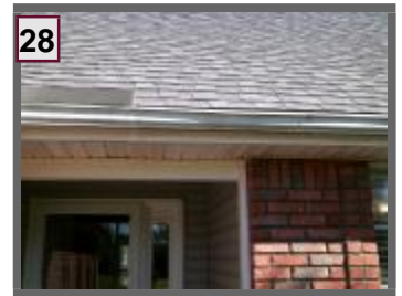
Gutters Damaged and lose.
