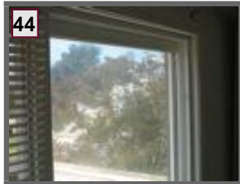
View of broken window glass at Master bedroom
